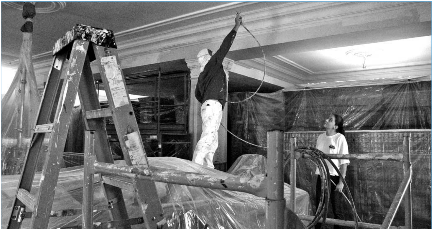
The library's paint scheme being restored to its original appearance. Also, although not pictured here, the heating and cooling system is being upgraded to better protect the important collections. These and other improvements should be completed in the next fiscal year.
