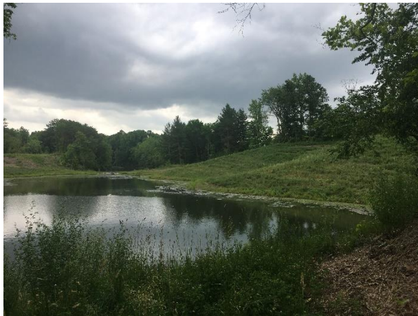
Completed reclamation of Whitney Pit western highwall. The highwall was backfilled to a 4:1 slope.
