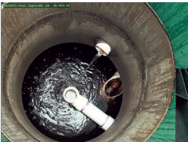
Pump discharge tank AFTER the repair of a High Strength Aerobic Treatment Unit using two Model 1200 pods metered forward flow average of 1,500 GPD.
