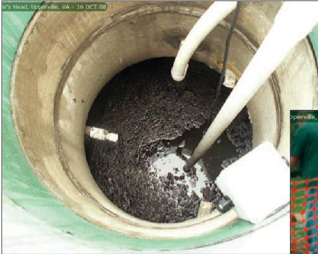
Pump discharge tank BEFORE the repair of a High Strength Aerobic Treatment Unit at a restaurant metered forward flow average of 1,500 GPD.
