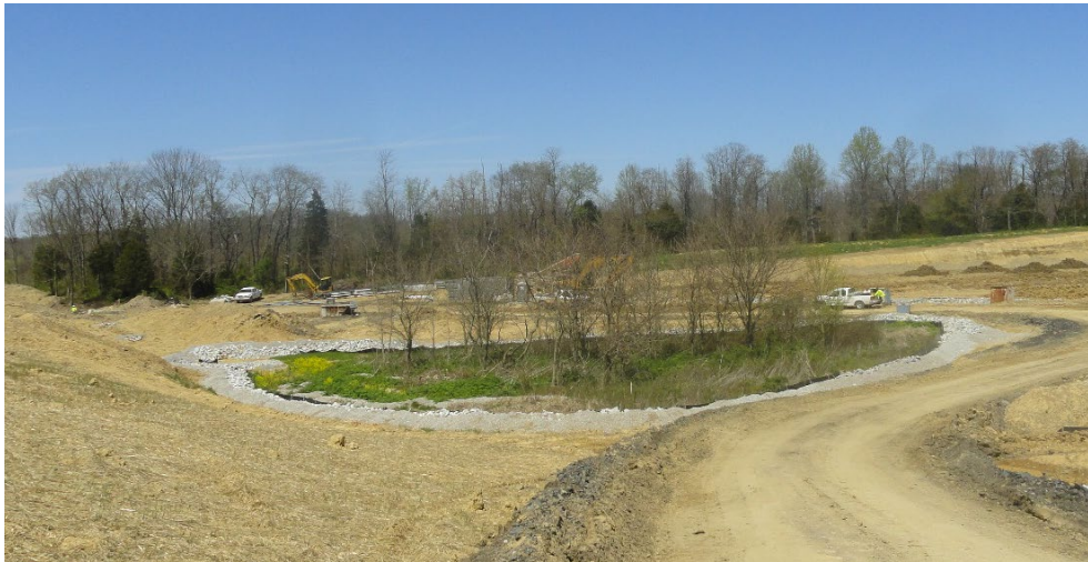
Rock ring protecting a large karst feature on the U.S. 50 North Vernon Bypass Photo credit INDOT
