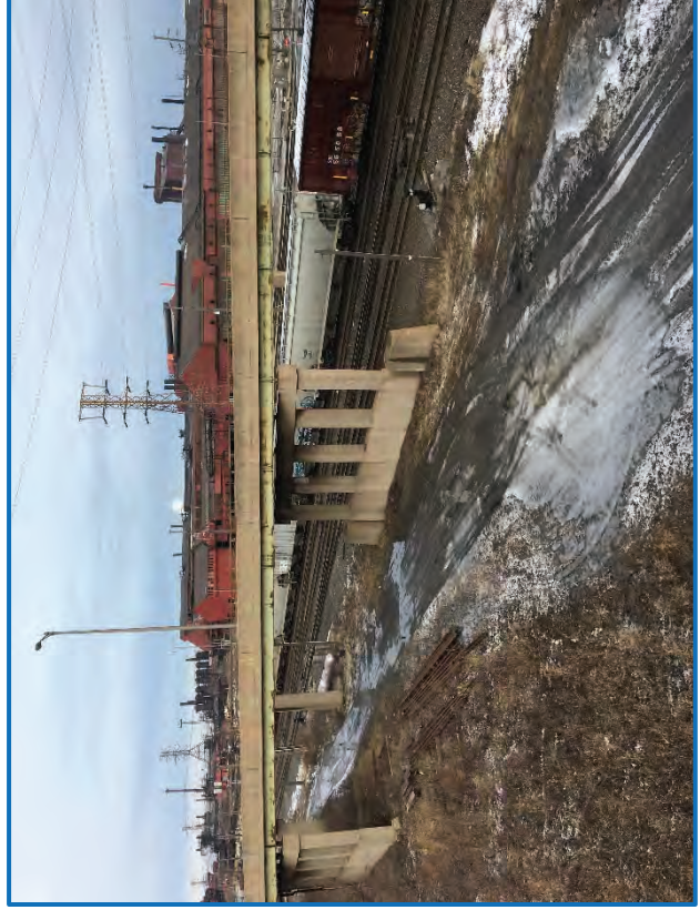
Photo 4 – View of the Ramp NEC bridge over railroad yard and service road facing northwest (2/14/2019).
