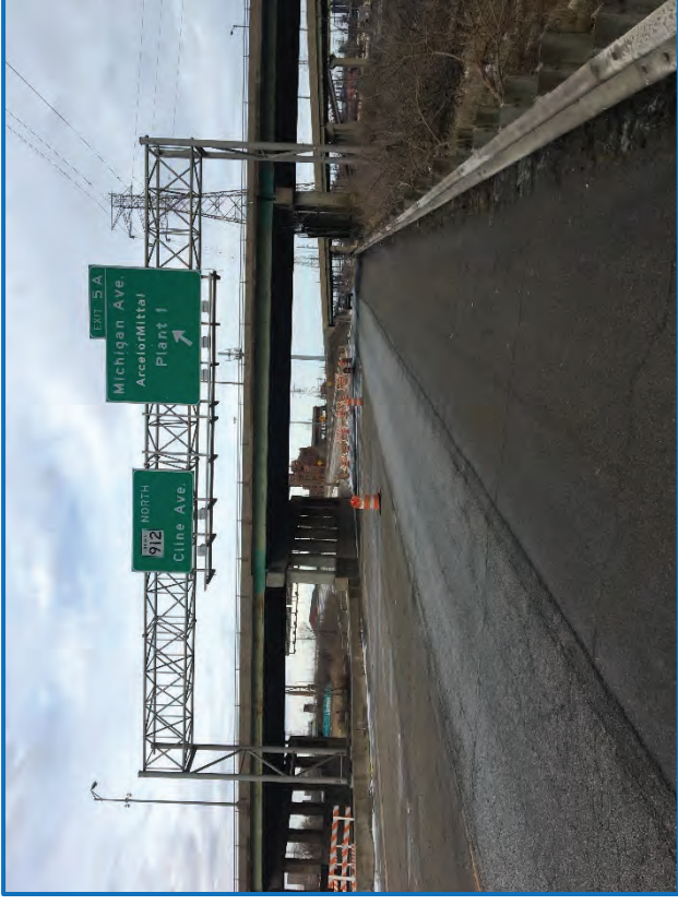
Photo 2 – View along westbound SR 912 of the Michigan Avenue Bridge over SR 912, railroad yard, and service road facing northwest (2/14/2019).
