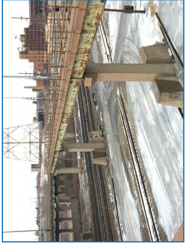
Photo 3 – View of pedestrian bridge over railroad yard and service road facing southwest (2/14/2019).
