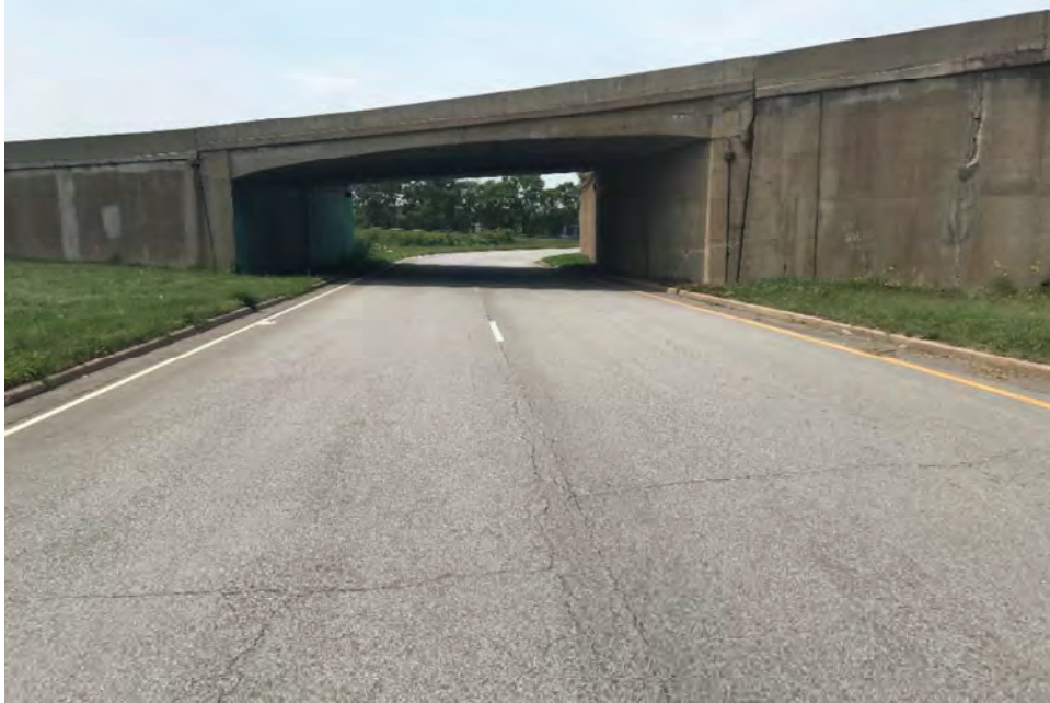
Photograph 3. Detailed view of the Ramp B over B bridge showing the structural slab top, taper of end walls, and evidence of previous patching attempts, looking west-southwest.
