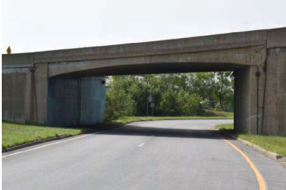
Photograph 2. Detailed view of the Ramp B over B bridge, looking west-southwest. Note taper of end walls from wider at top to narrower at bottom.
