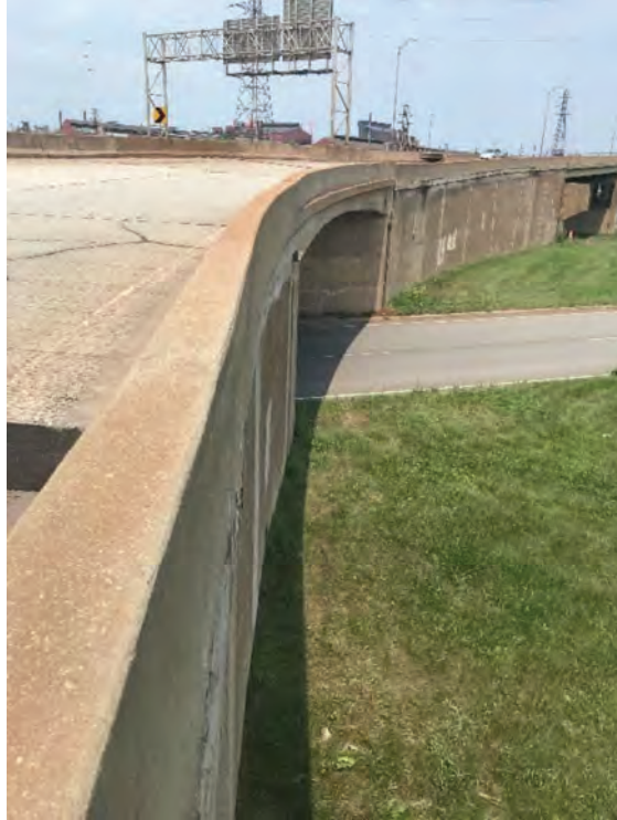
Photograph 9. Overview of the Ramp B over B bridge showing a large piece of concrete protruding, looking north from the deck approach.
