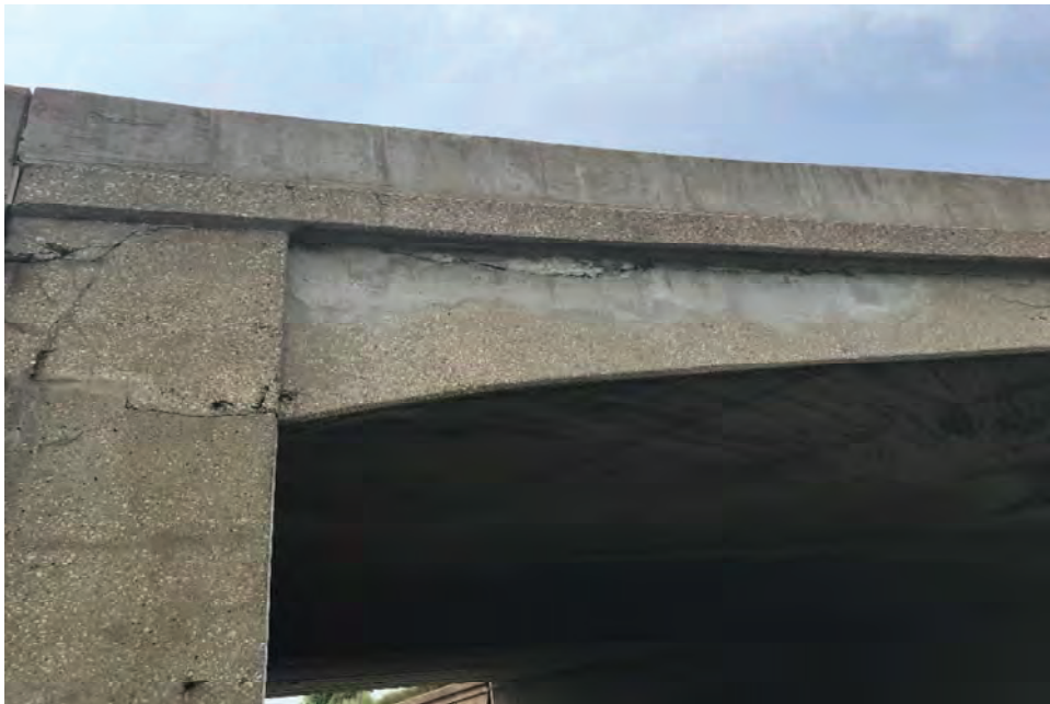
Photograph 4. Detailed view of the Ramp B over B bridge showing cracking, chipping, and patching on the arch, looking west-southwest. Note the previous patching attempts are already failing.
