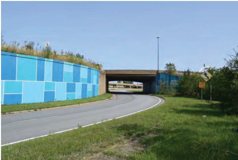
Photograph 8. View of the Ramp B over B bridge from Block Avenue showing INDOT mitigation signs, including arrows and "Stay Right" signage to address horizontal sight stopping distance issues, looking north-northeast.
