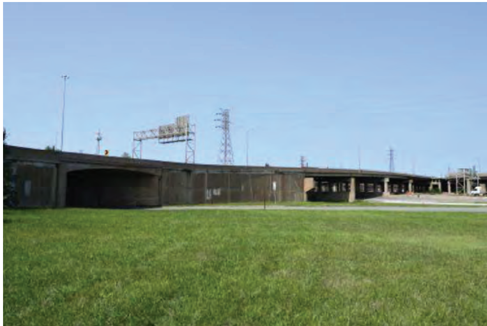
Photograph 10. Overview of Ramp B over B and the Michigan Avenue Overpass. Photo taken looking north from Block Avenue/Commonwealth Avenue.
