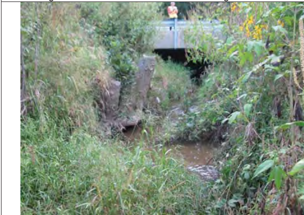
7. Looking southeast on the west side of the bridge, looking upstream of Wells Ditch.
