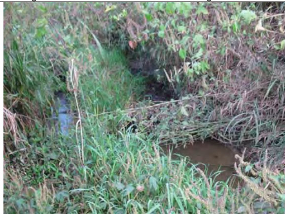
8. Looking northwest on the west side of the bridge, downstream in Wells Ditch. Note in-stream vegetation.
