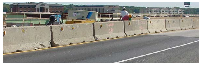
Figure 7-2 Temporary Traffic Barriers
