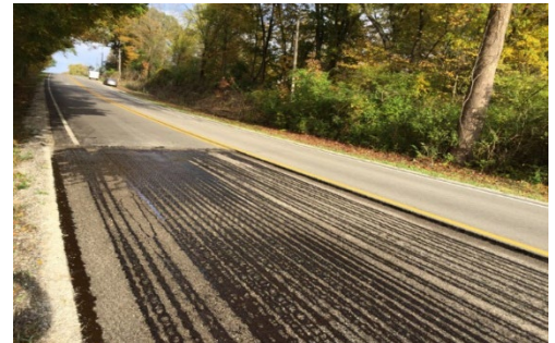
Figure 4-8 Poor Tack Coat Application
