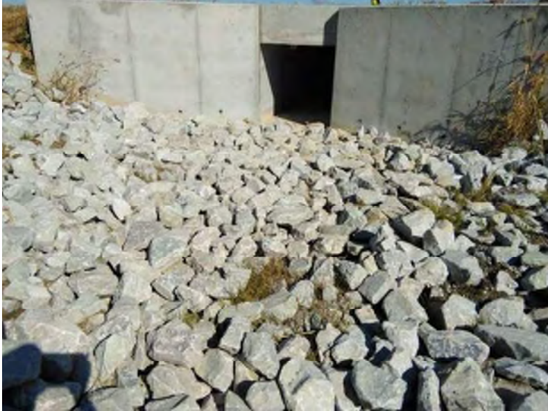
PP-13; Looking north at the culvert that carries UNT 2 from the south side of SR 244 (9-29-2020).
