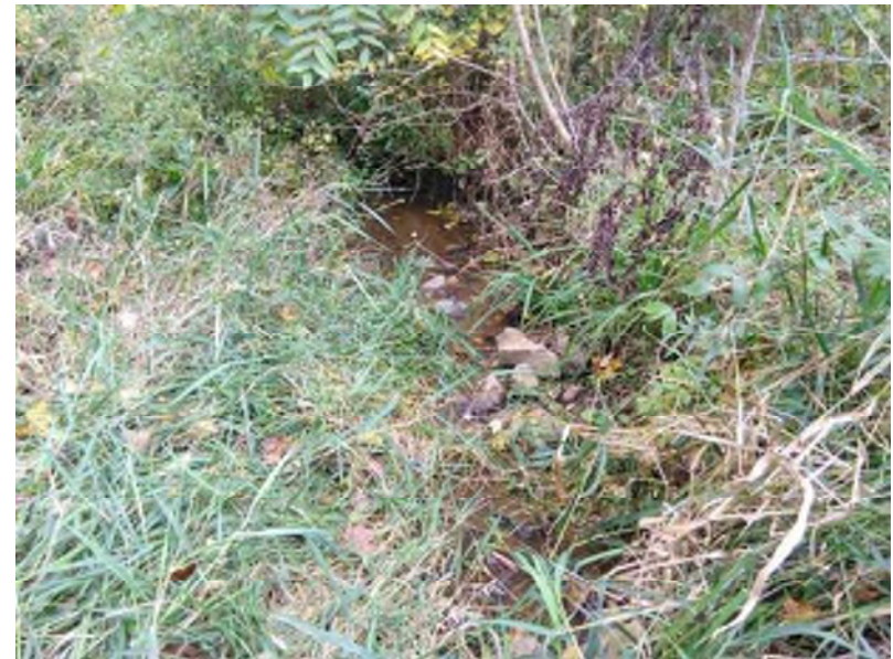
PP-37; Looking south, downstream at UNT 4 from the culvert on the south side of SR 244 (9-29-2020).
