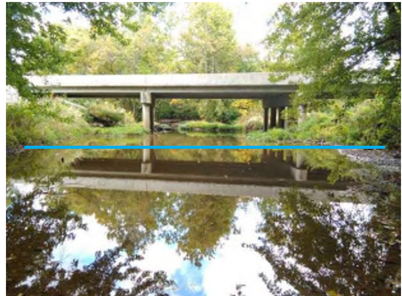
PP-24; Looking north, upstream at Conns Creek and the SR 244 bridge (9-29-2020). OHWM at 39.497219, -85.642751
