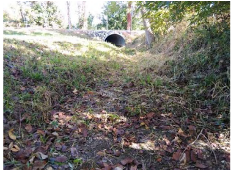
PP-16; Looking north at RSD 2 and the culvert under SR 244 from the southern study area boundary (9-29-2020).
