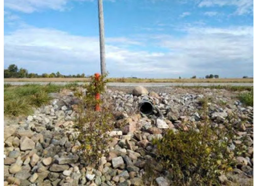
PP-39; Looking north at the SR 244 culvert along the agriculture drainage swale (9-30-2020).
