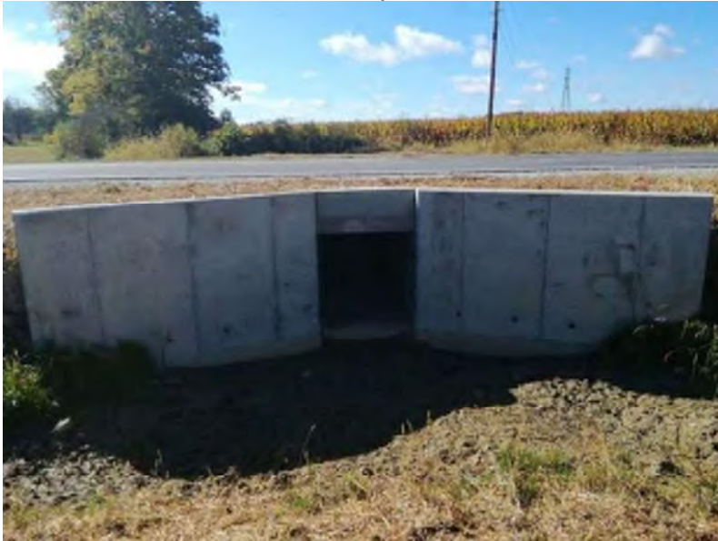
PP-9; Looking south at the culvert where UNT 2 begins from the north side of SR 244 (9-29-2020).
