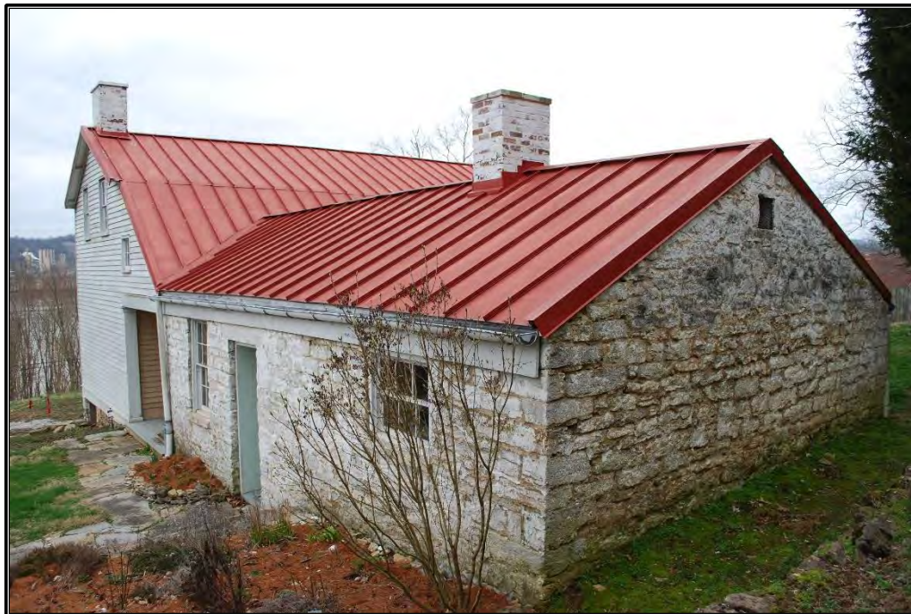
Figure B-7. Rear (north) and east elevation, facing south. Visible is a metal replacement roof.
