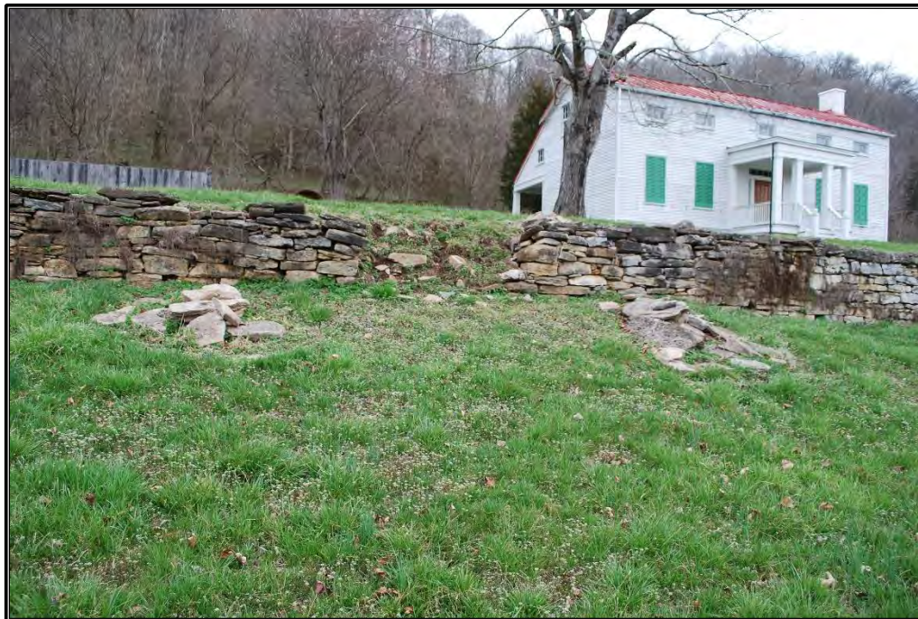
Figure B-19. View of retaining wall (Resource G) south of residence, with visible erosion, facing north.
