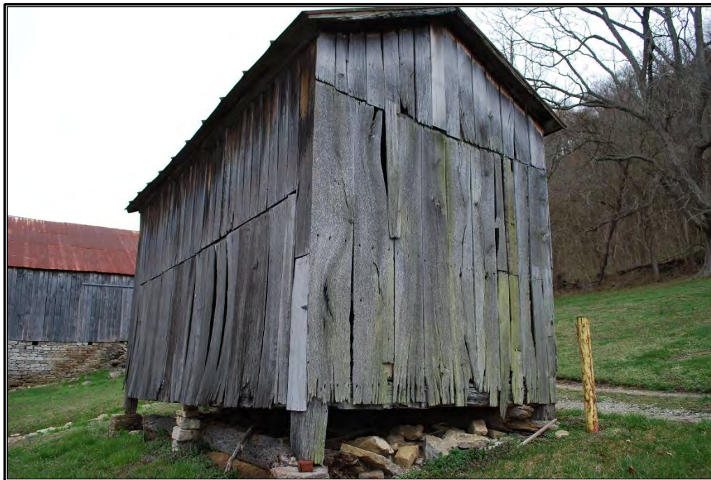
Figure B-11. East and south elevations of granary (Resource B), facing west.
