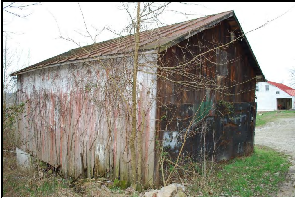
Figure B-15. North and east elevations of carriage house/buggy shop (Resource D), facing south.
