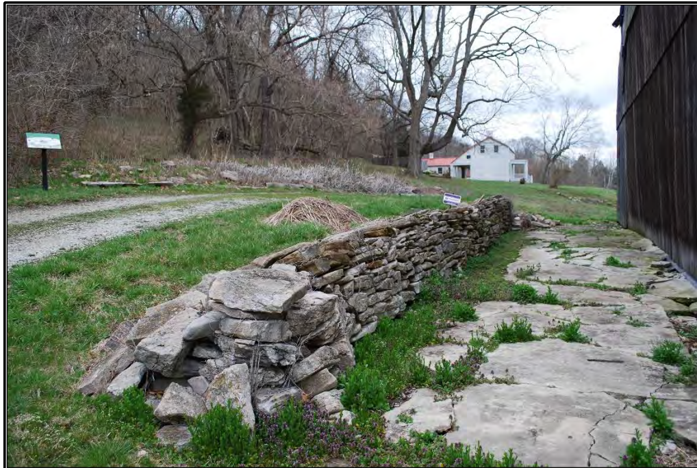
Figure B-17. View of dry-laid stone wall (Resource F) north of hay press barn, facing northeast.
