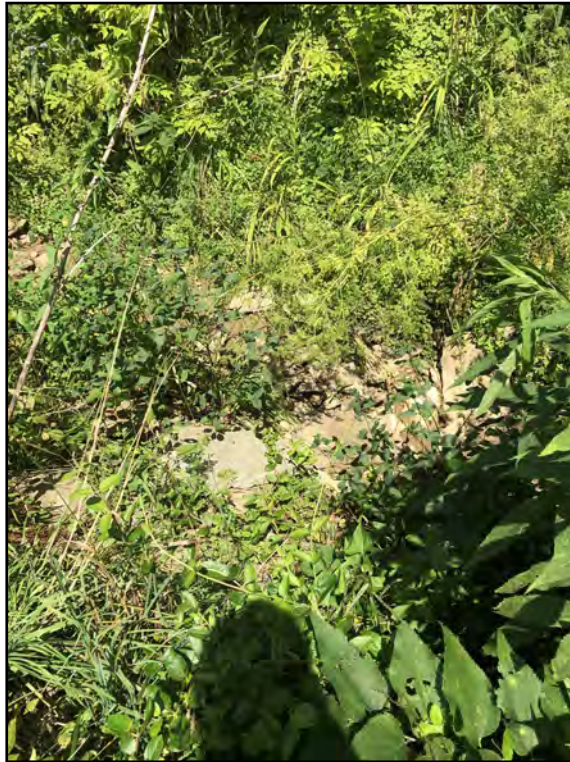
Photo 9: Bank on the southeast side of the culvert. Channel is saturated but no surface water is present.
