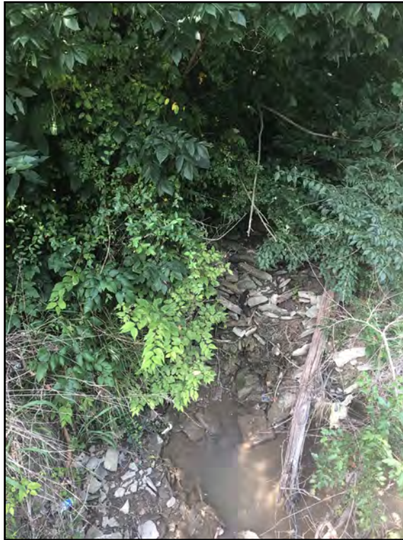
Photo 3: Looking over the northwest side of the culvert at the pool caused by Stream 1 (UNT to Ohio River).
