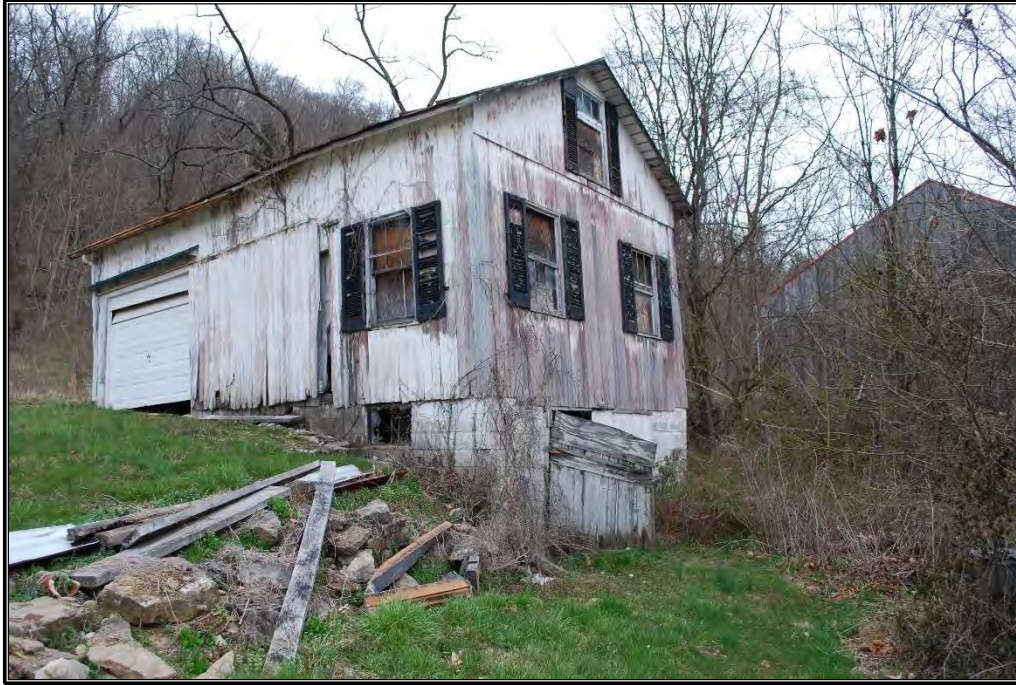
Figure B-14. South and west elevations of carriage house/buggy shop (Resource D), facing north.
