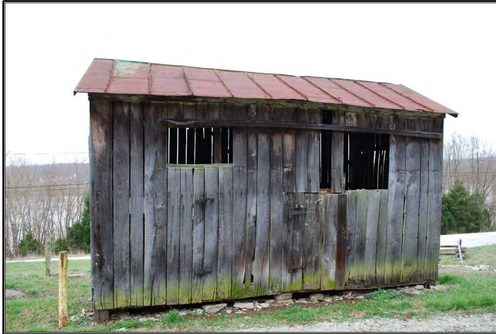
Figure B-12. North elevation of granary (Resource B), facing southeast. Deterioration of cladding is visible.
