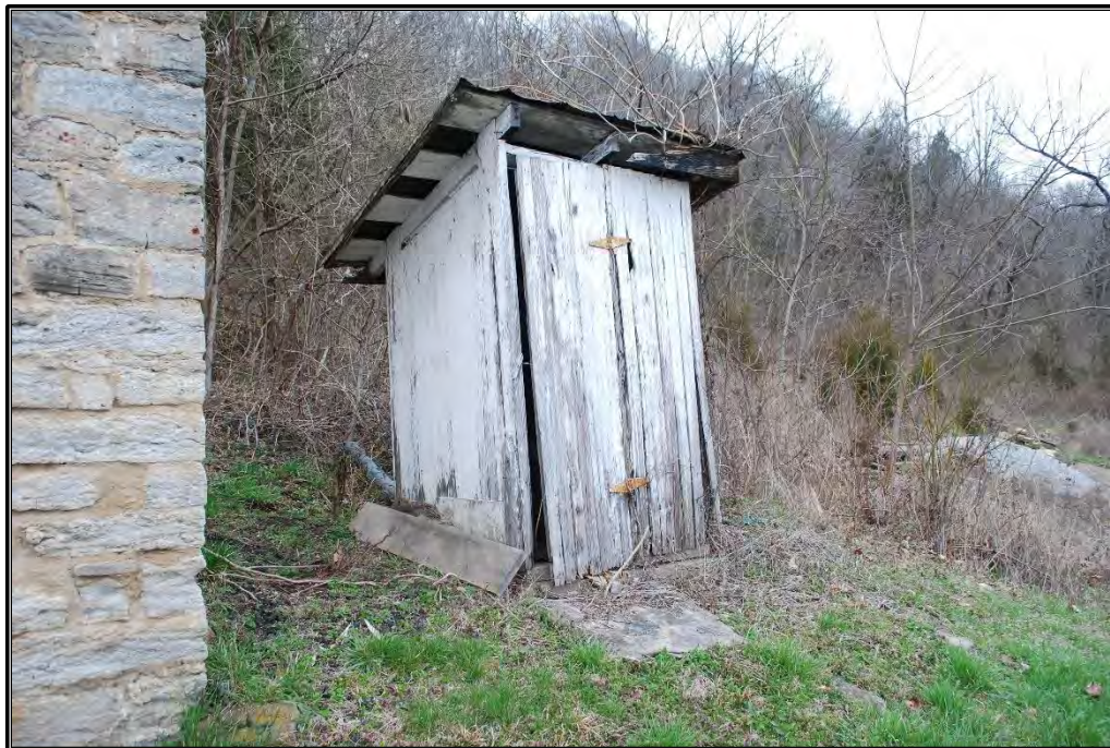
Figure B-13. South and west elevations of privy (Resource C), facing north.
