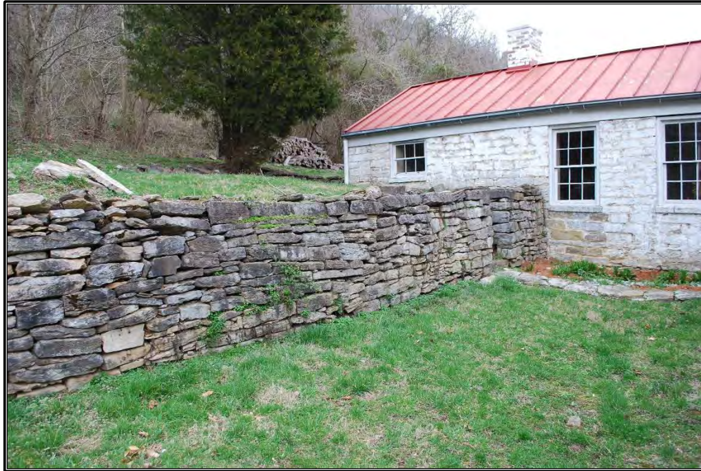
Figure B-18. View of dry-laid stone wall (Resource F) north of residence, facing north.
