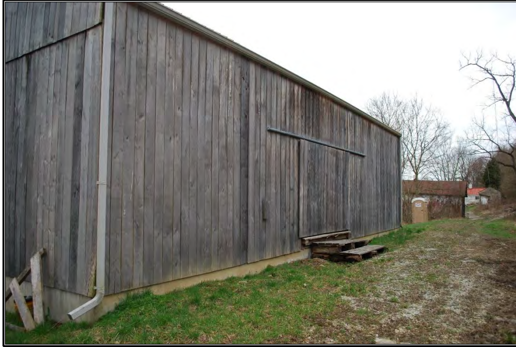
Figure B-28. Wood frame barn (Resource O), north and east elevations, facing south.
