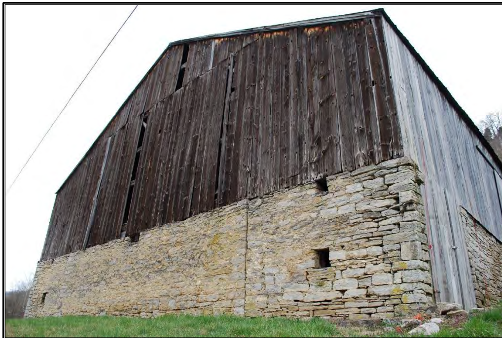
Figure B-9. South and east elevations of hay press barn (Resource A), facing west.
