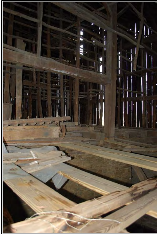
Figure B-10. View of interior of hay press barn (Resource A), facing southeast. Poles for tobacco barn conversion are visible.
