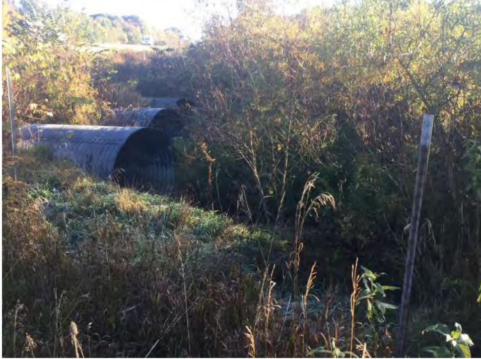
Photo 13: Facing east—view of downstream end of structures carrying Prairie Ditch beneath US 24.
