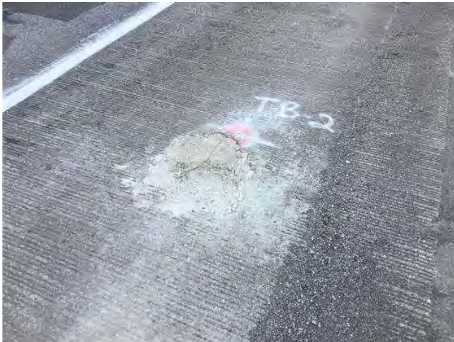
PHOTO 6 Condition Description Excess Concrete in the West Shoulder
