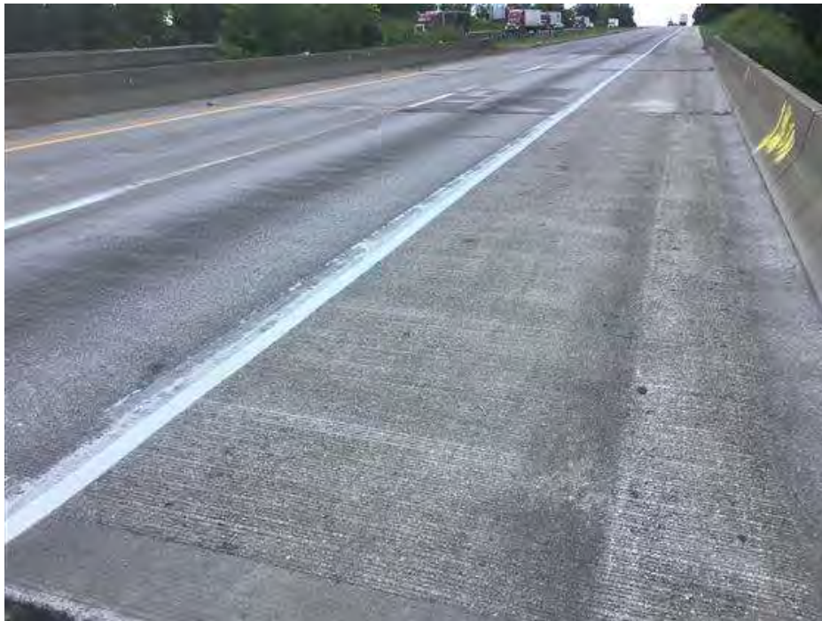
PHOTO 8 Condition Description Deck facing South
