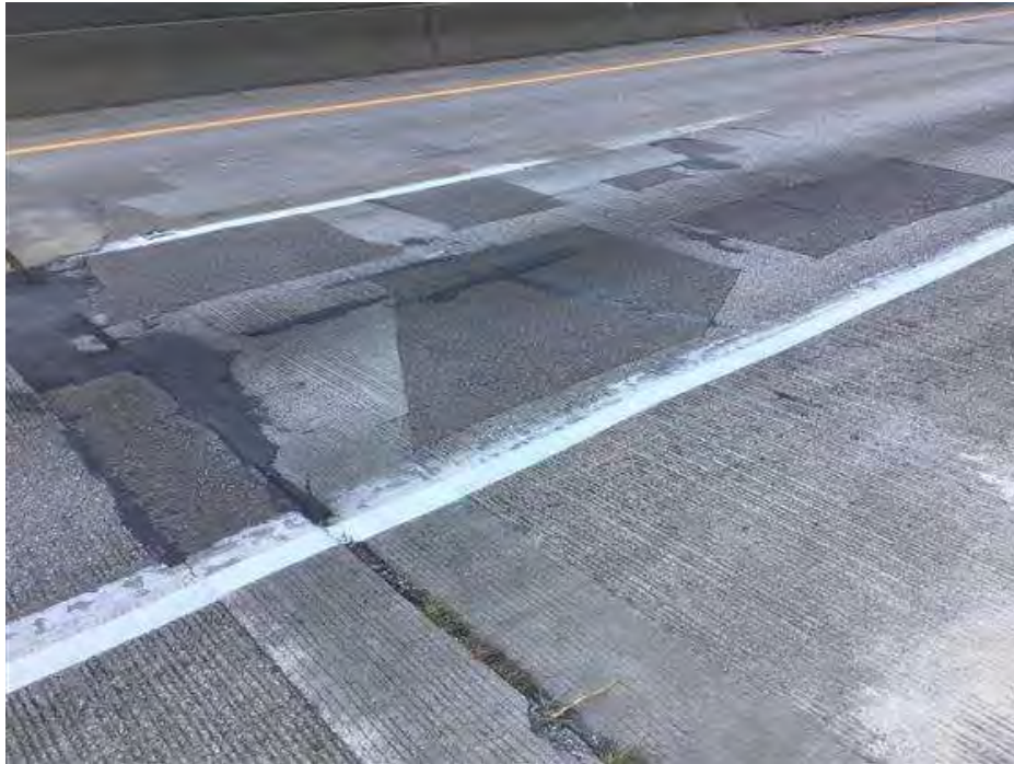
PHOTO 5 Condition Description Patches over Span B
