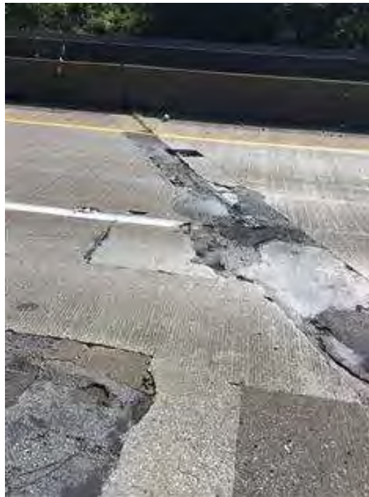
PHOTO 8 Condition, Other, Maintenance - Bridge Description Joint 3 facing east.
