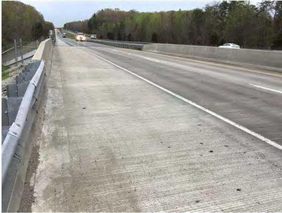
PHOTO 3 Condition Description Roadway south.
