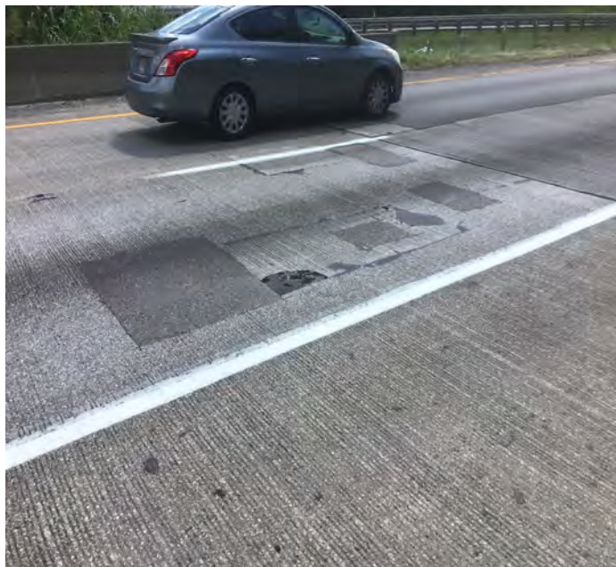
PHOTO 1 Description Patches on South end of the Deck
