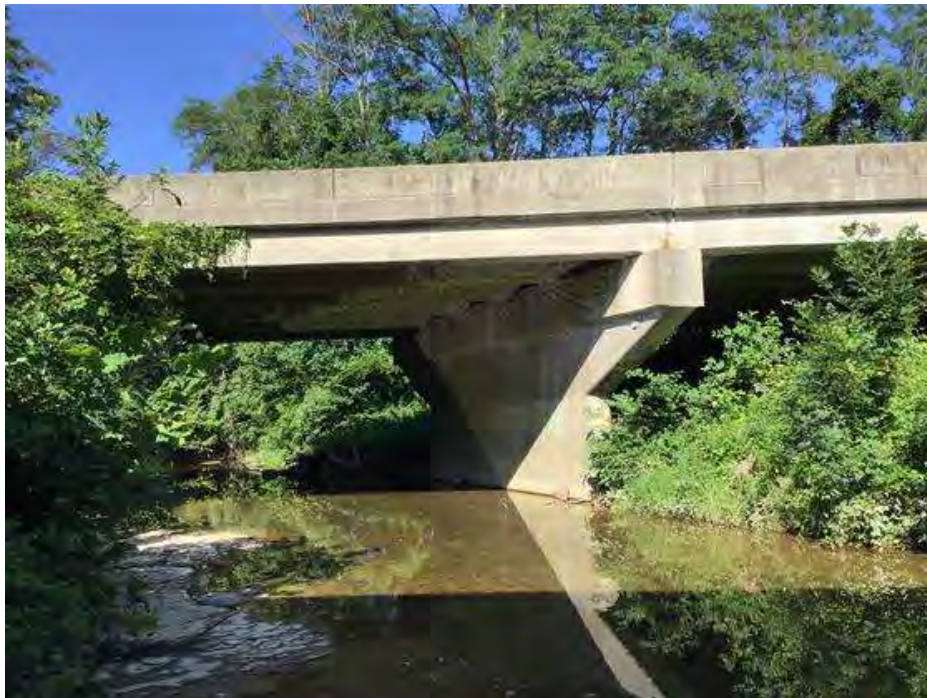
PHOTO 2 Elevation, Condition Description East side.
