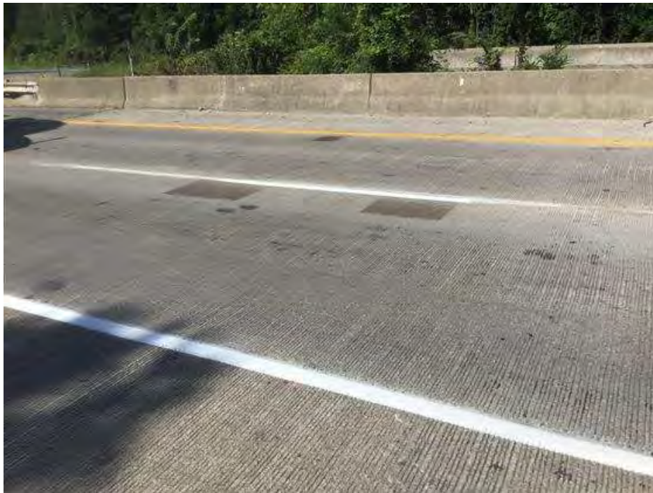
PHOTO 4 Condition Description Patches over Span A
