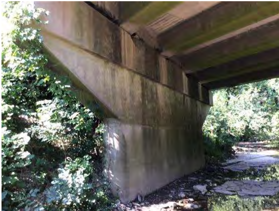
PHOTO 16 Condition Description Pier 2 north side.
