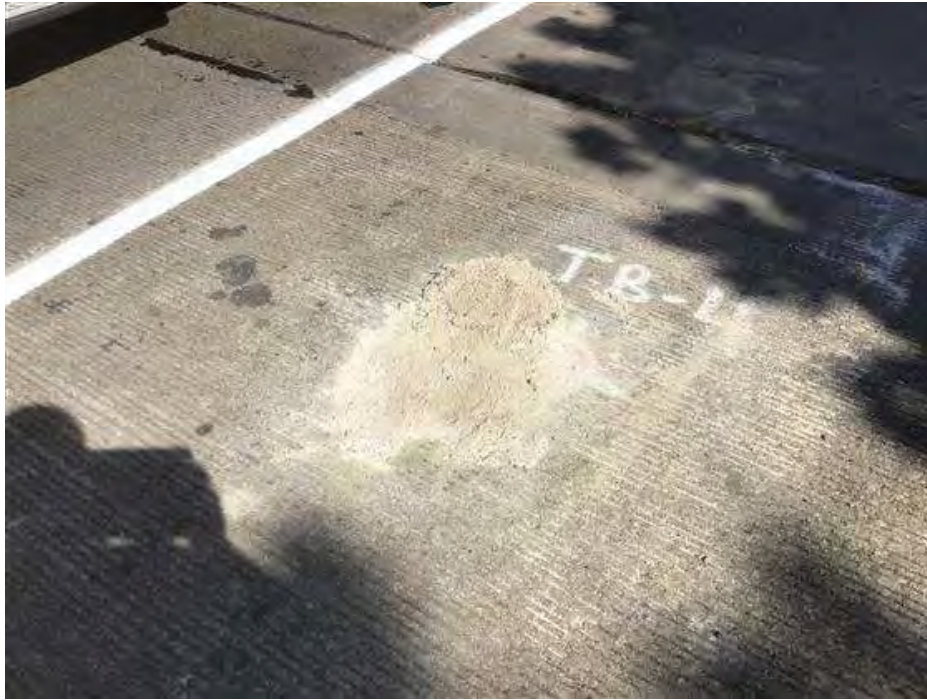
PHOTO 7 Condition Description Excess Concrete on the East Shoulder near Joint #2
