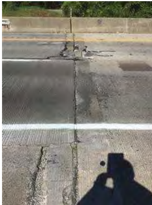
PHOTO 2 Condition, Maintenance - Bridge Description South Joint facing West 2' X 2' and 3' X 1' Spall
