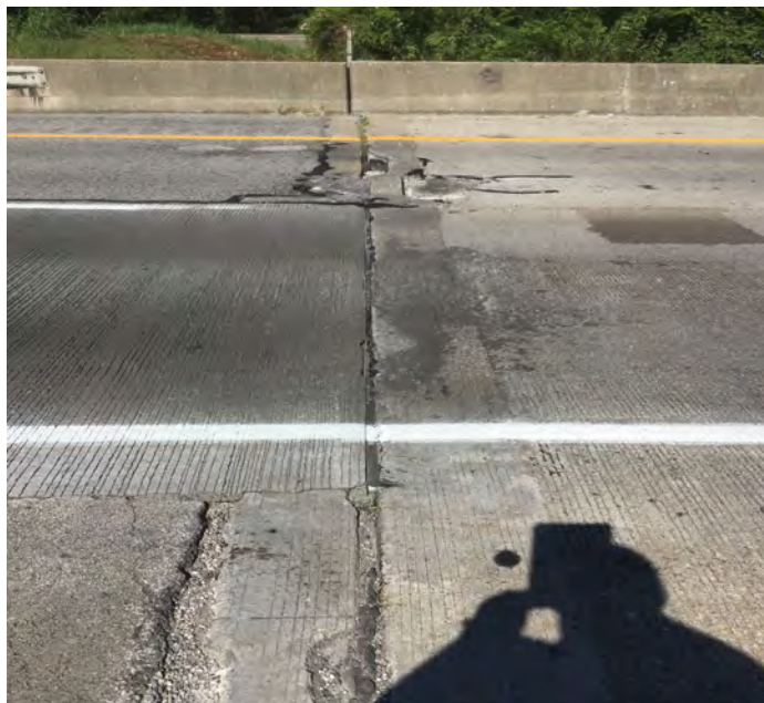
PHOTO 1 Description South Joint facing West 2' X 2' and 3' X 1' Spall
