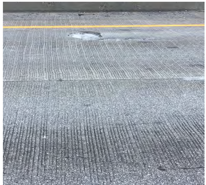
PHOTO 2 Description 3' X 3' Spall in the Passing Lane over Span B
