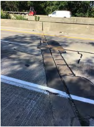
File Description Joint 2 facing west. File Type Category Condition, Maintenance - Bridge, Other
