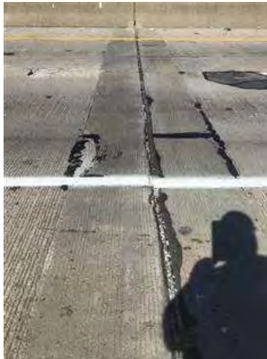
PHOTO 8 Condition Description Joint over Pier #3 facing West
