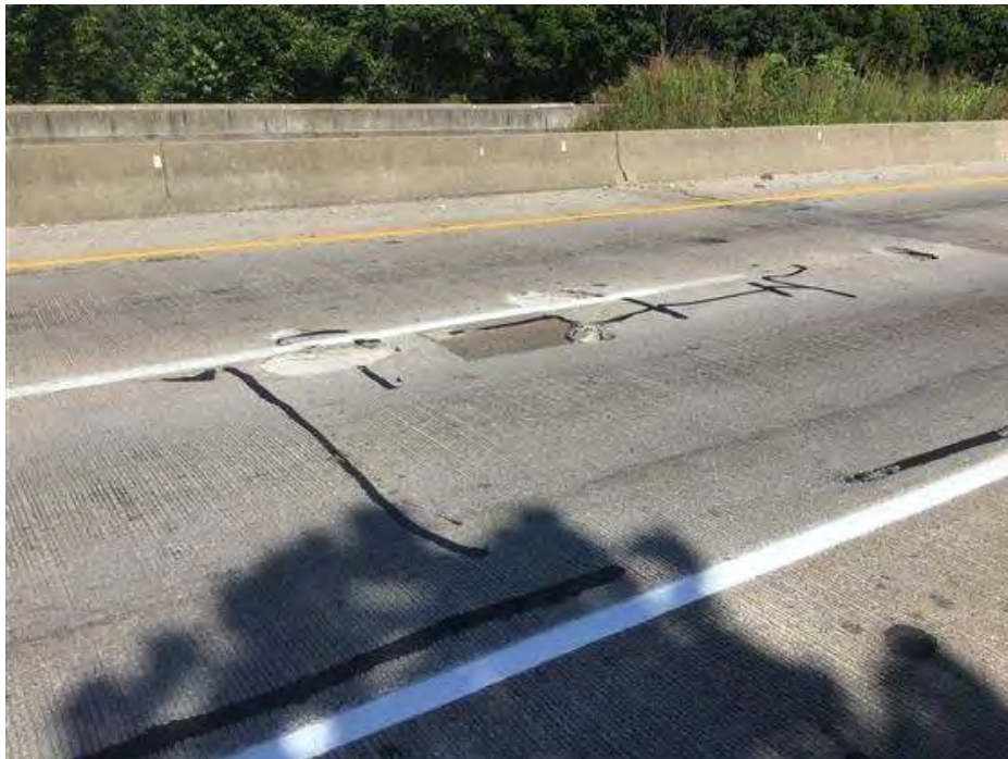
PHOTO 6 Condition, Maintenance - Bridge Description 4 Spalls (two 2' X 2' and two 1' X 1') over Span B
