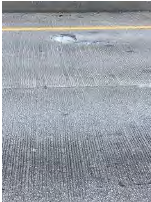
PHOTO 4 Condition, Maintenance - Bridge Description 3' X 3' Spall in the Passing Lane over Span B
