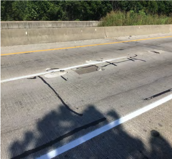
PHOTO 3 Description 4 Spalls (two 2' X 2' and two 1' X 1') over Span B
