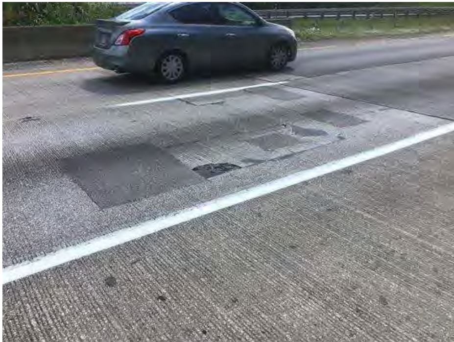
PHOTO 2 Condition Description Patches on South end of the Deck
