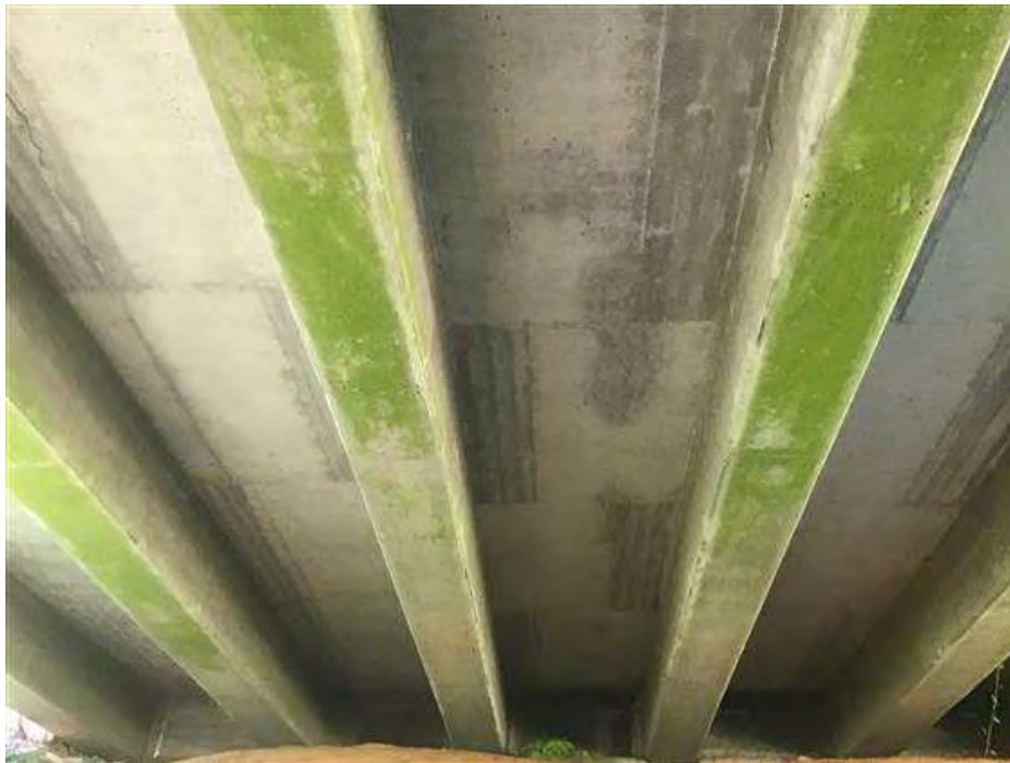
PHOTO 12 Condition Description Underside Span A and Abutment #1 facing South
