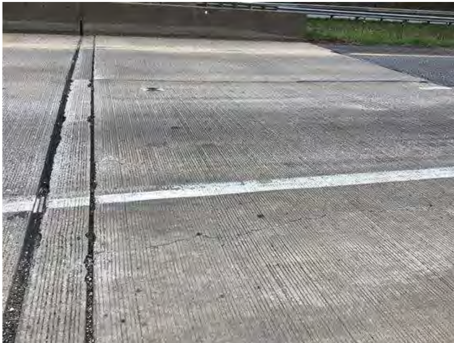
PHOTO 6 Condition Description North joint and approach slab.
