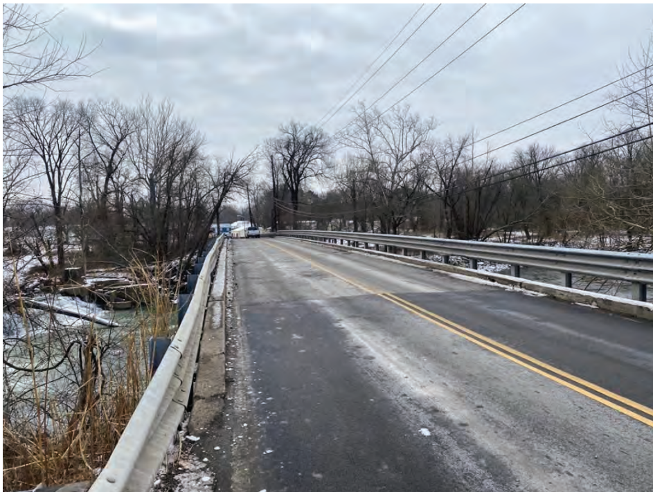
Photo 28. View of Blackiston Mill Road facing south from the north approach of Bridge No. 51
