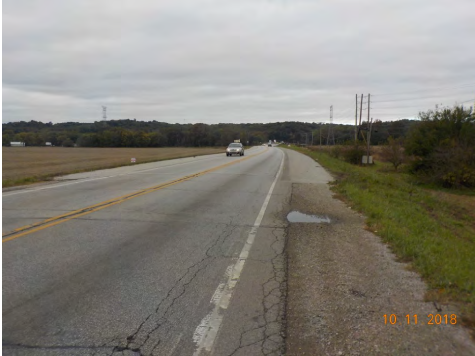
F 89. View of SR 39 showing the area of milling and repaving, looking northwest.
