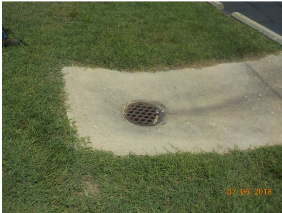
F 61. View of a storm drain in front of the CVS at SR 39 and Randolph Street, looking north.
