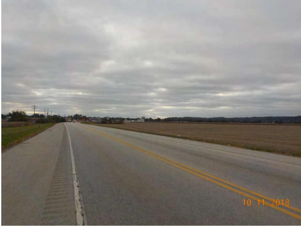
F 90. View of SR 39 showing the area of milling and repaving, looking southeast.
