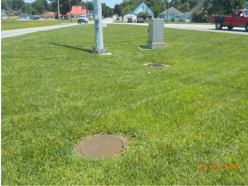
F 86. View of the traffic island at the intersection of SR 39 and Morgan Street, looking east.
