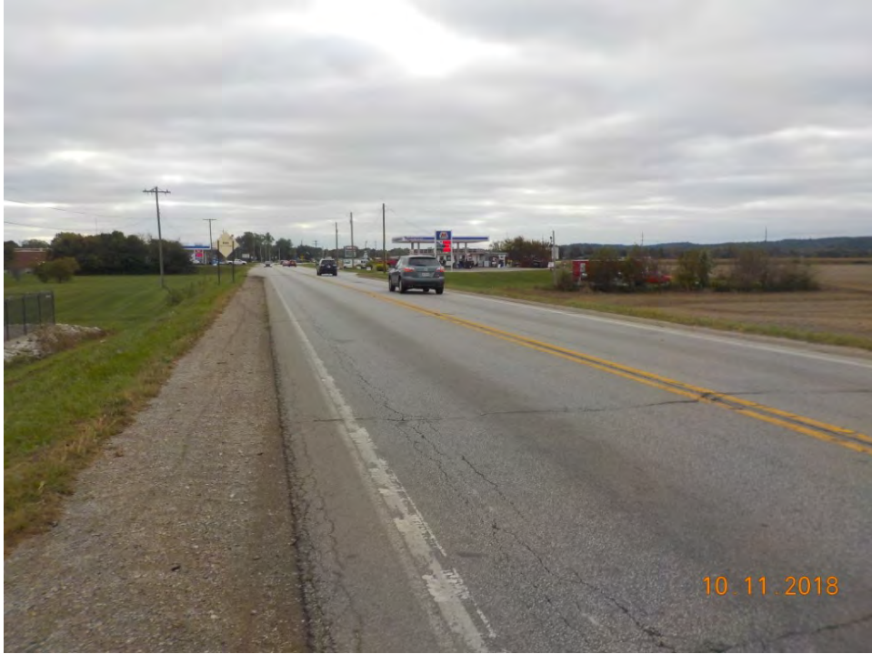
F 88. View of SR 39 showing the area of milling and repaving, looking southeast.
