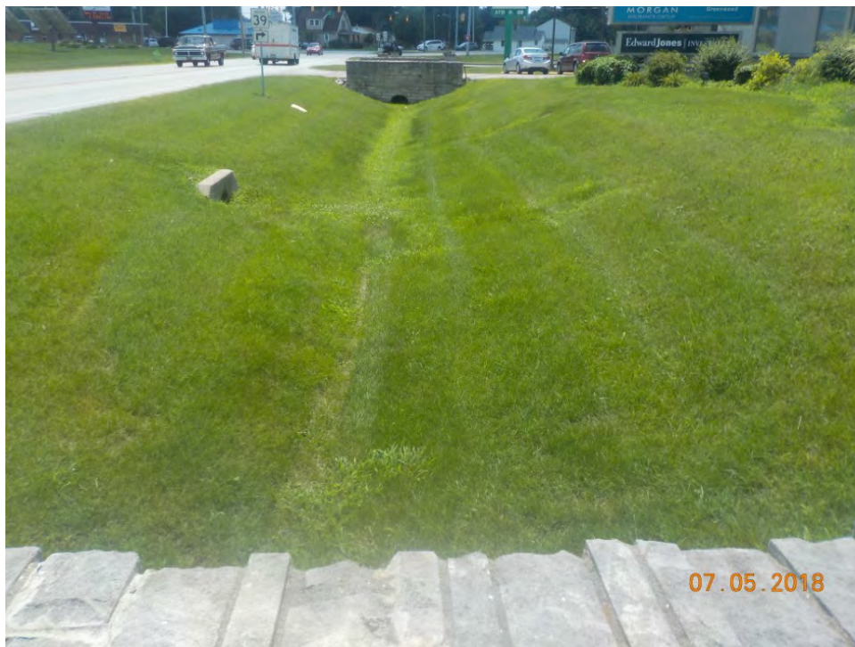
F 43. View of the west side of the project area at the intersection of SR 39 and Morton Avenue showing the area disturbed by a roadside ditch and culverts, looking southeast.
