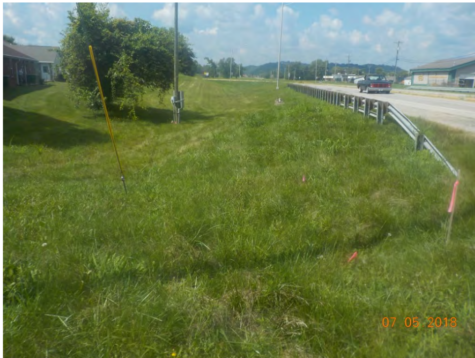
F 25. View of the south end of the project area disturbed by the construction of the SR 37 and SR 39 interchange, looking southwest.
