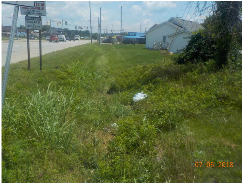
F 45. View of the east side of the project area at the intersection of SR 39, Morton Avenue, and Harriett street showing the area disturbed by a roadside ditch, looking northeast.
