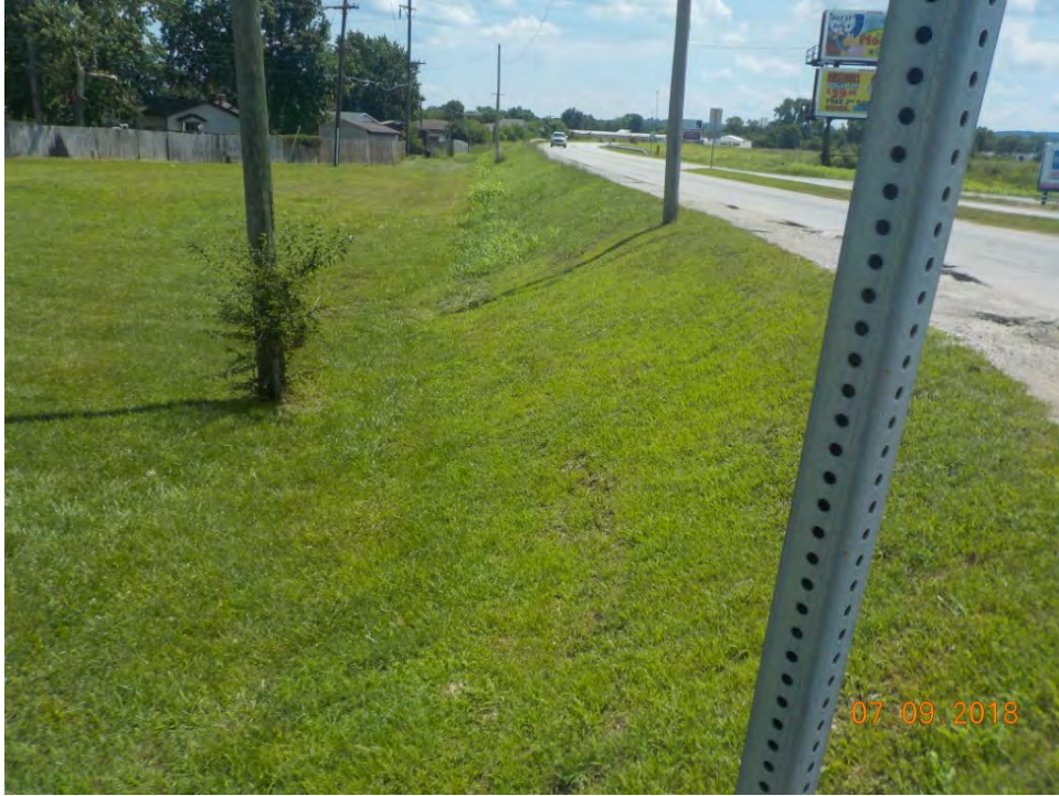
F 72. View of the east side of the project area at Morgan Street showing disturbance by the road grade and shallow ditch, looking southeast along SR 39.
