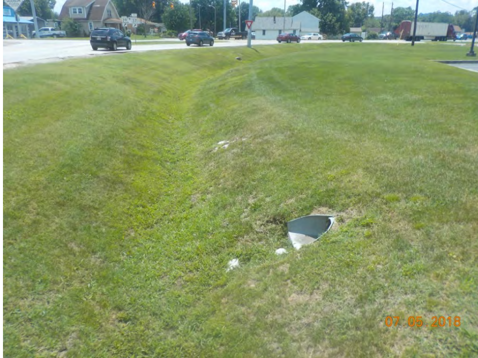
F 42. View of the west side of the project area at the intersection of SR 39 and Morton Avenue showing the area disturbed by a roadside ditch and culverts, looking south.
