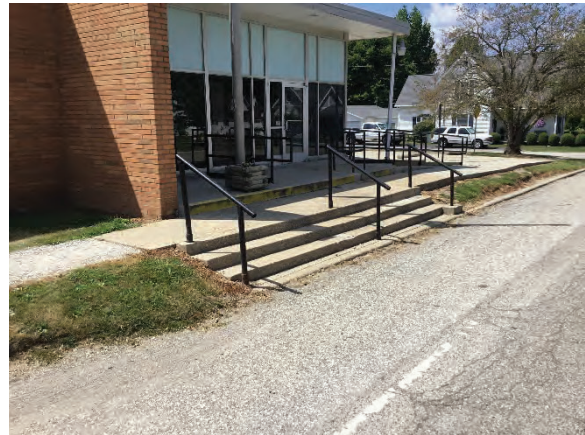
Figure 2: Looking southwest at the Waveland Post Office steps that are proposed to be retained.
