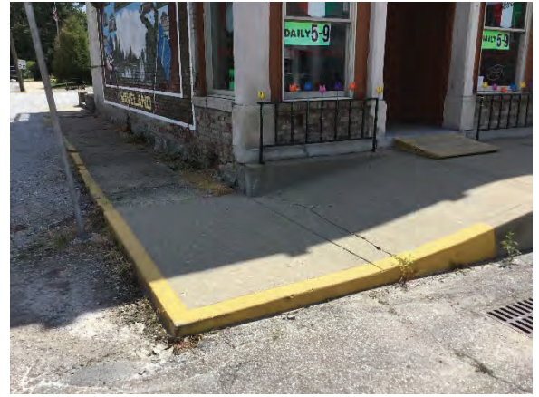
Figure 16: Looking southeast at the non-contributing (post 1985) concrete sidewalk ramp in front of the Union Block.
