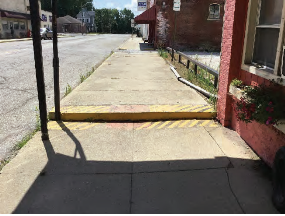
Figure 15: Looking south at the non-contributing (post 1985) sidewalk step along the west side of Cross Street.
