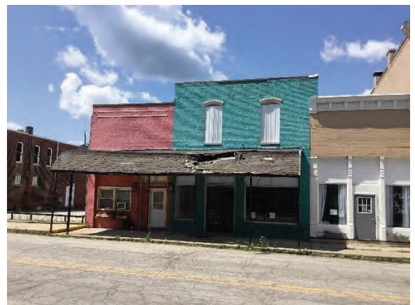
Figure 14: Looking southwest at the non-contributing awning in front of the commercial building at 224 Cross Street.
