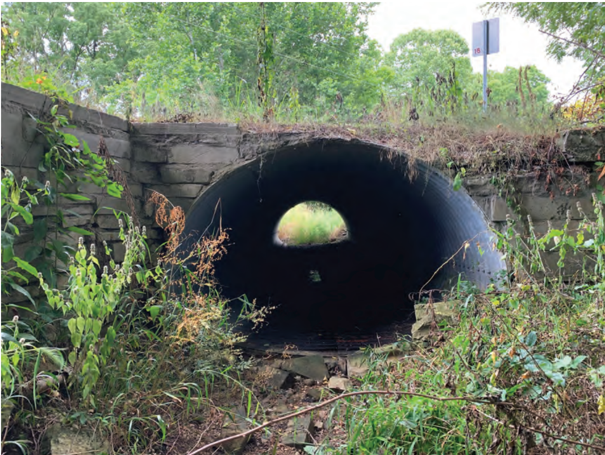
4. View of UNT 1 to Leatherwood Creek culvert inlet under SR 58 facing southwest
