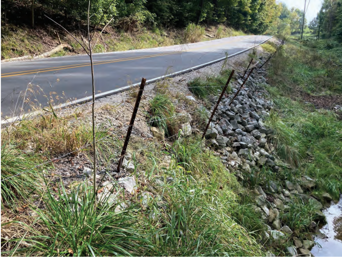
9. Looking east at SR 58 and failing embankment
