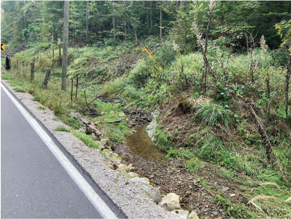
7. Looking southeast at shoulder, embankment, and stream along westbound SR 58
