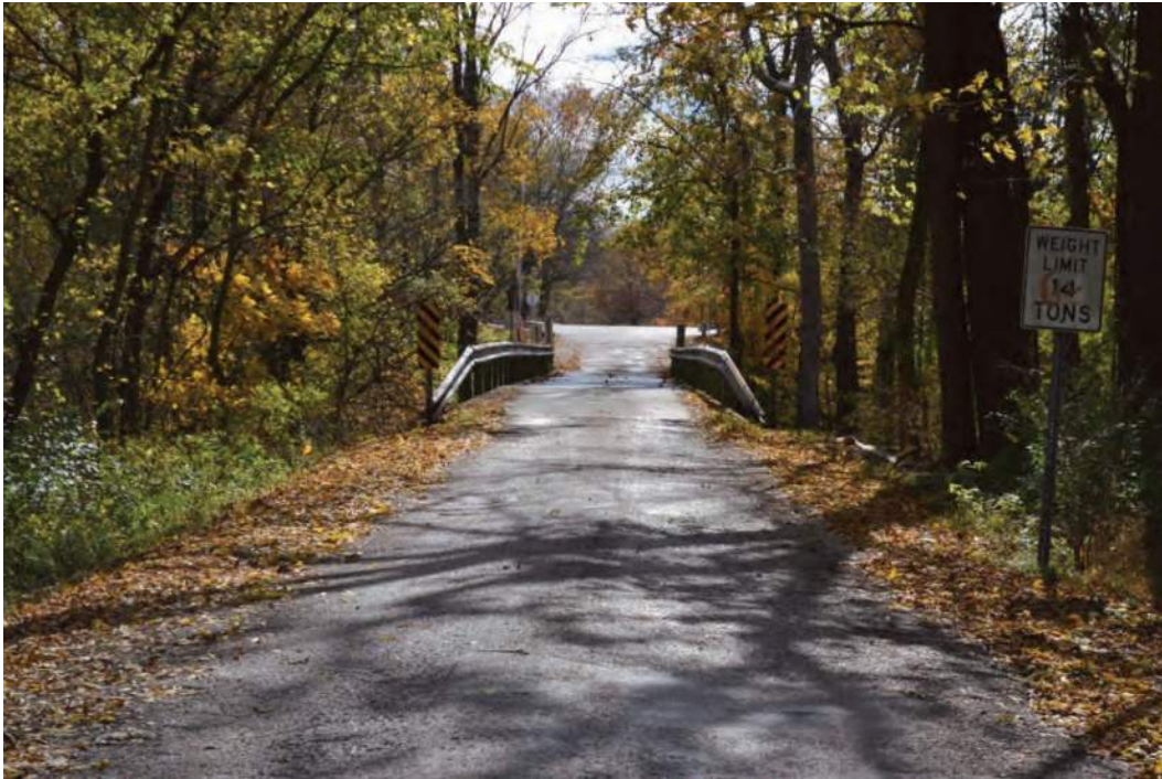
Photo 1. View along Brickyard Road taken from the northern side of Boggs Creek and showing Martin County Bridge No. 58, facing southeast
