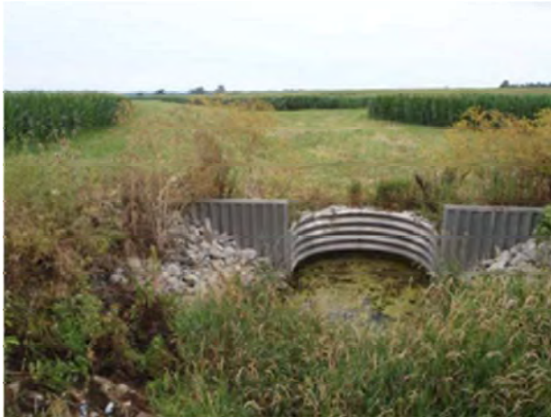
1. Looking north from the structure at the UNT to Panther Creek and agricultural field
