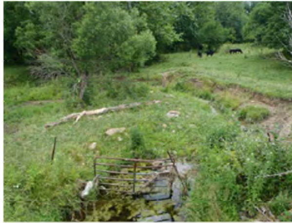
5. Looking south from the structure at the UNT to Panther Creek and adjacent property
