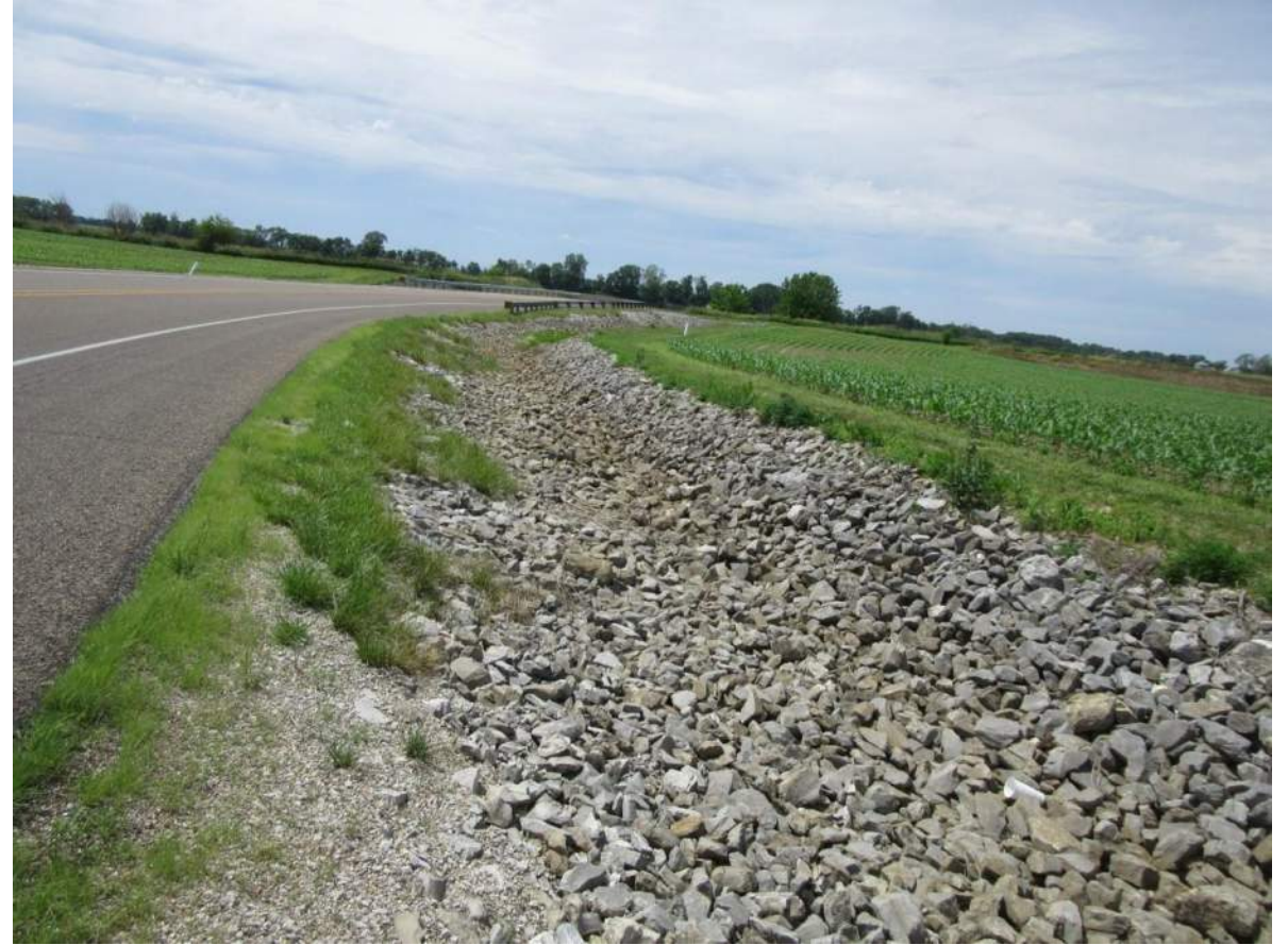
18. Looking northeast up ditch line on the east side of SR 42. Photo taken 6/12/19.
