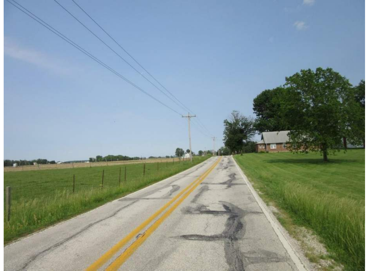
54. Looking east up SR 42 from Structure No. 33 (not pictured). Right-of-way is anticipated at this location to replace the structure. Photo taken 6/3/19.
