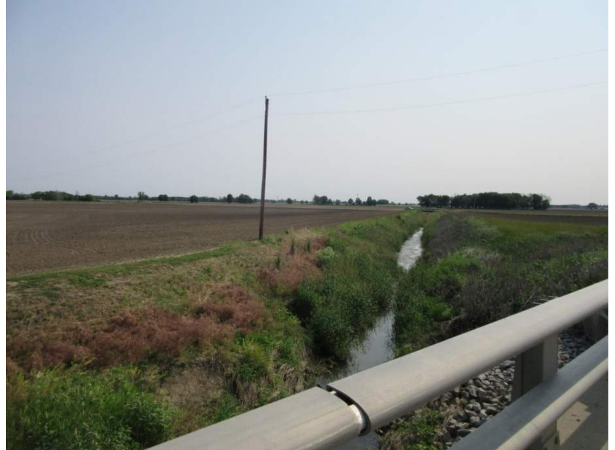
88. Looking northeast up UNT 2 to Lake Ditch from an exempted structure. Photo taken 6/3/19.
