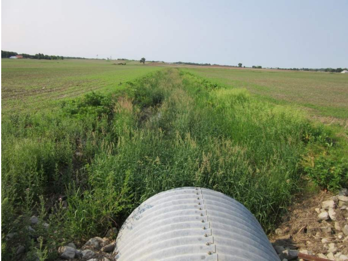
97. Looking south down UNT 1 to Lake Ditch and Structure No. 45 from SR 42. Photo taken 6/3/19.
