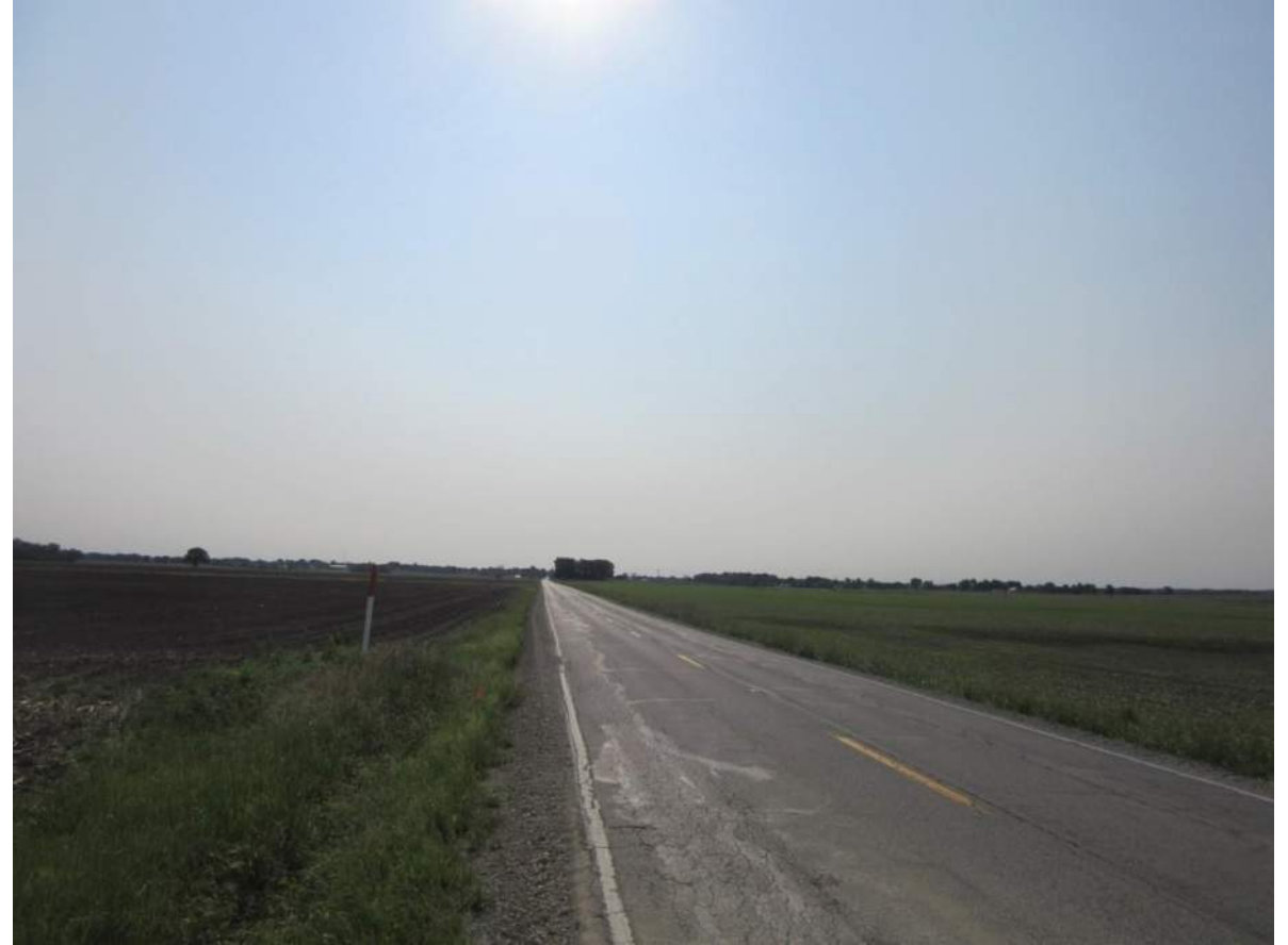
96. Looking east down SR 42 from the intersection of SR 42 and N. Allen Rd. Photo taken 6/3/19.
