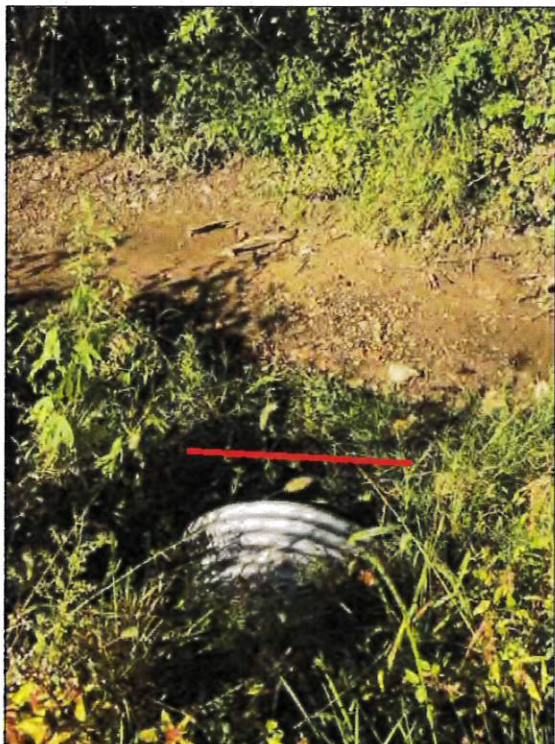
Picture 80—UNT2 to White Creek corrugated metal pipe outlet and OHRM; west view; 9-23-22.
