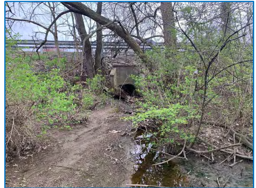
Photo 6 – View of SR 22, the outfall of pipe arch culvert Structure CV 022-027-49.42, and UNT 1 to Jefferson Ditch, facing west (04-22-20).
