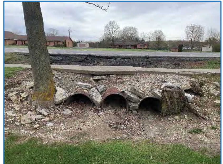
Photo 8 – View facing west of triple corrugated metal pipe inlets that drain into a grassy swale to Jefferson Ditch, INDOT Structure No. CV 022-027-49.72 (4-23-2020).
