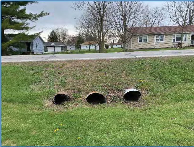
Photo 5 – View facing east of triple corrugated metal pipe outlets that drain into a grassy swale to Jefferson Ditch, INDOT Structure No. CV 022-027-49.72 (4-23-2020).
