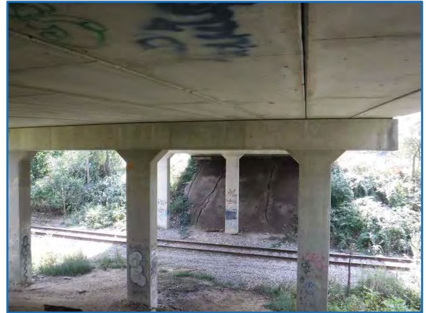
Photo 2 – View facing southeast of the underside of the SR 22 bridge over the CERA, INDOT Structure No. 022-27-02130 A (10-1-2019).
