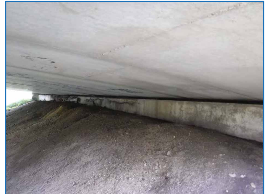
Photo 4 – View facing northwest of the north abutment of INDOT Structure No. 022-27-02130 A (10-1-2019).
