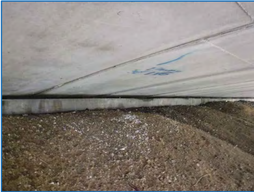
Photo 1 – View facing southwest of the south abutment of the SR 22 bridge over the Central Railroad of Indianapolis (CERA), INDOT Structure No. 022-27-02130 A (10-1-2019).
