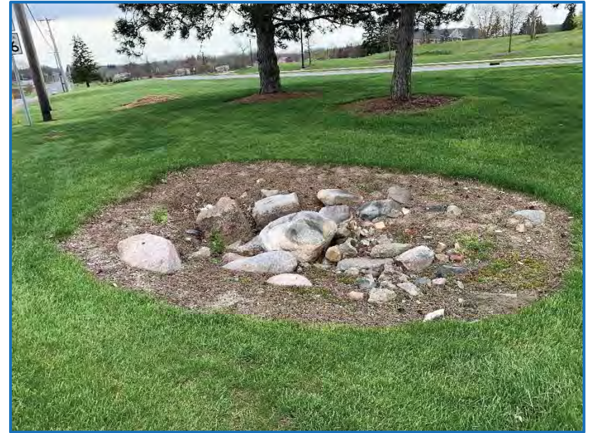
Photo 6 – View facing south of rock covered stormwater inlet along the west side of SR 22 near Taylor University (4-23-2020).
