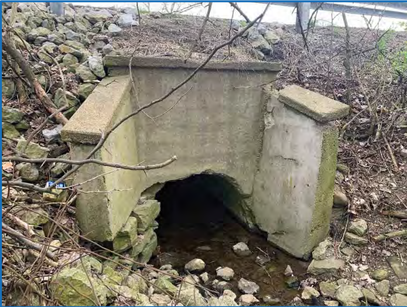
Photo 5 – View facing west of concrete stormwater outfall to Jefferson Ditch, INDOT Structure No. CV 022-027-49.42 (4-23-2020).
