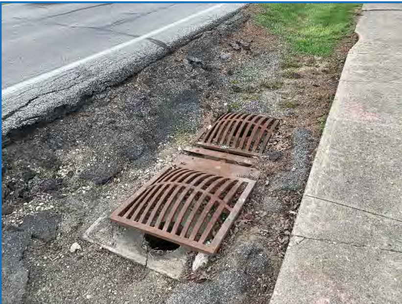
Photo 7 – View facing south of dual stormwater inlet grates that drain into a grassy swale to Jefferson Ditch, INDOT Structure No. CV 022-027-49.72 (4-23-2020).
