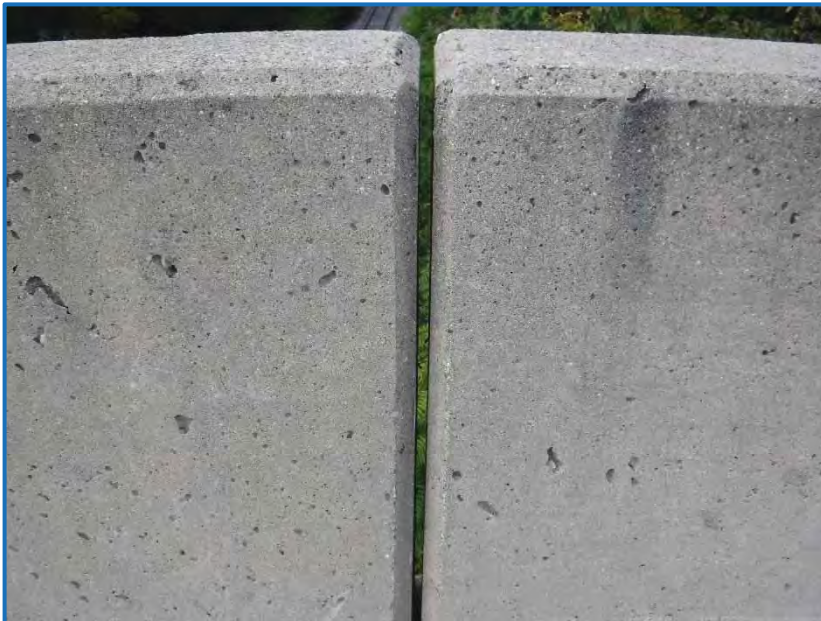
Photo 3 – View facing west of crevice along the west side of INDOT Structure No. 022-27-02130 A (10-1-2019).
