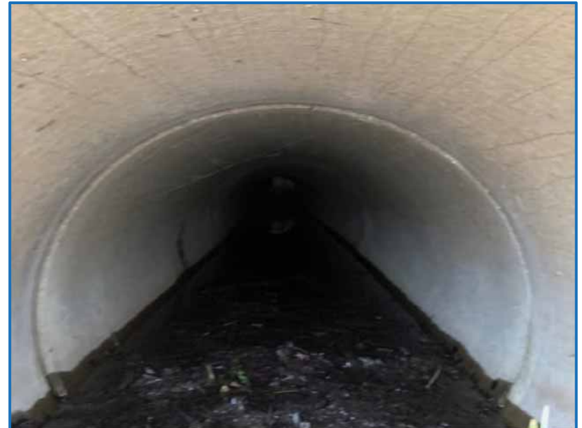
Photo 6 – View facing west of the interior of a stormwater outfall that drains into a wetland along the east side of SR 22 near Taylor University (4-23-2020).
