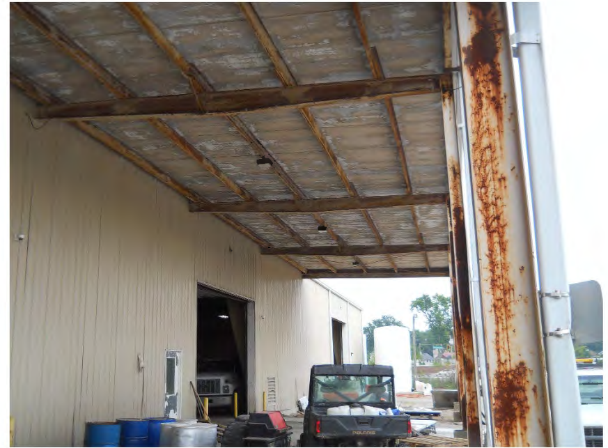
City garage – south canopy steel condition
