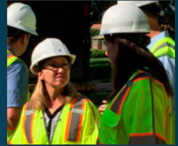
Analysts Jennifer Sisson and Crystal Barrett visit a water utility construction site.
